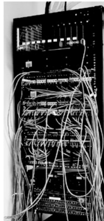
A Networking Substation in a Small Server Room with Poorly Managed Patch Cords
